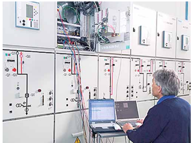
Fig. 2/34 Protection engineer at work
