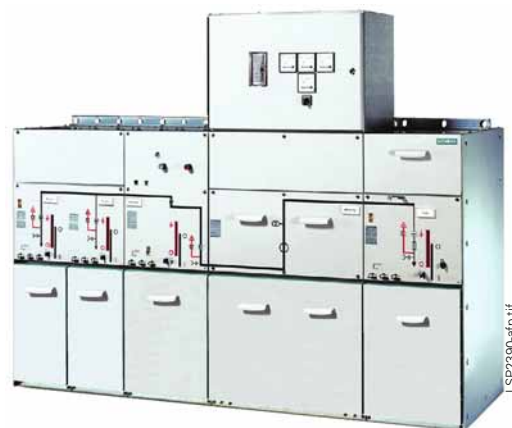
Fig. 5/13 Application in distribution switchgear
