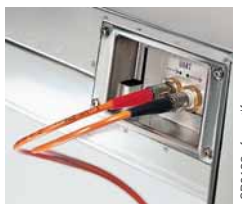
Fig. 5/36 View from below showing system interface (SCADA) with FO connection (for remote communications)
