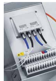
Fig. 6/7 Communication interfaces in a sloped case in a surface- mounting housing
