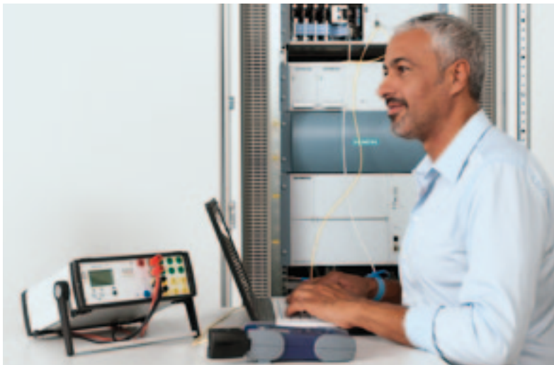
Commissioning of the SWT 3000
