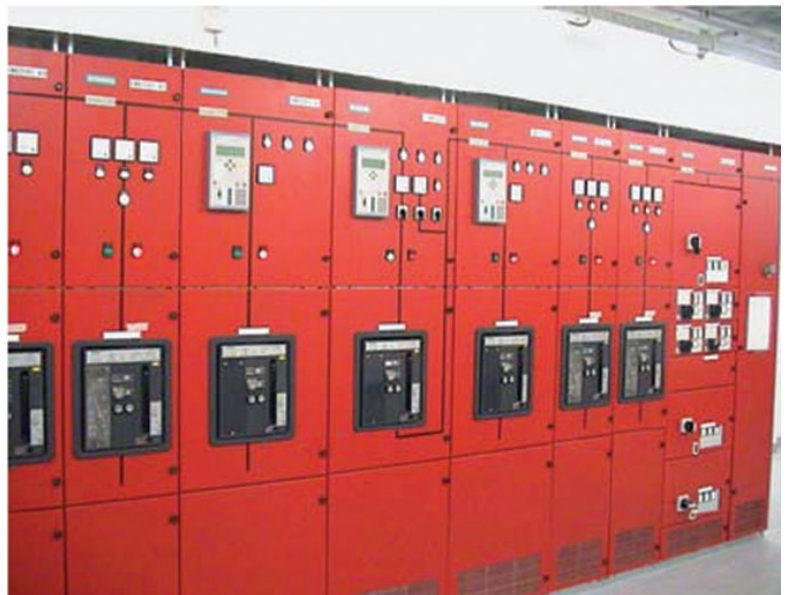
Fig. 1 SIVACON 400 V, with 7SJ62-protected and controlled circuit-breakers
