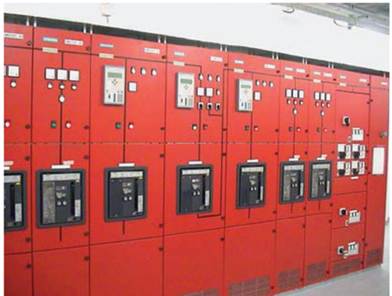
Fig. 1 SIVACON 400 V, with 7SJ62-protected and controlled circuit-breakers
