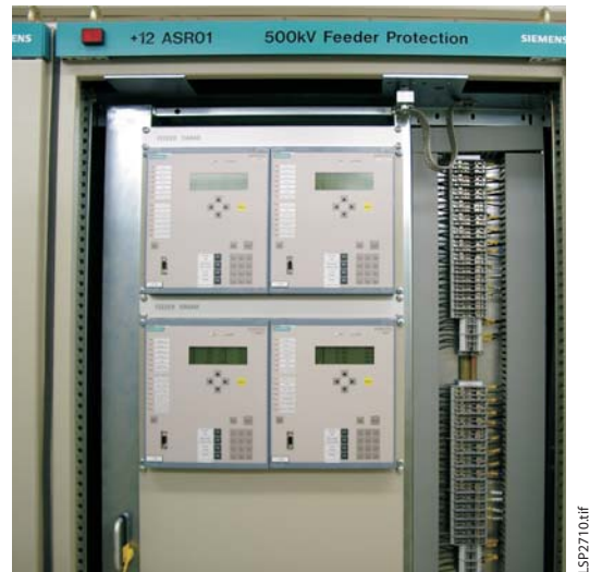
Fig. 3 Main and backup protection 7SD52 and 7SA522
