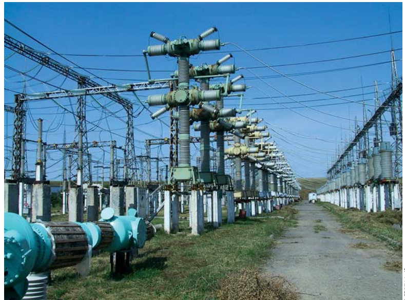
Fig. 1 Substation in Kazakhstan
