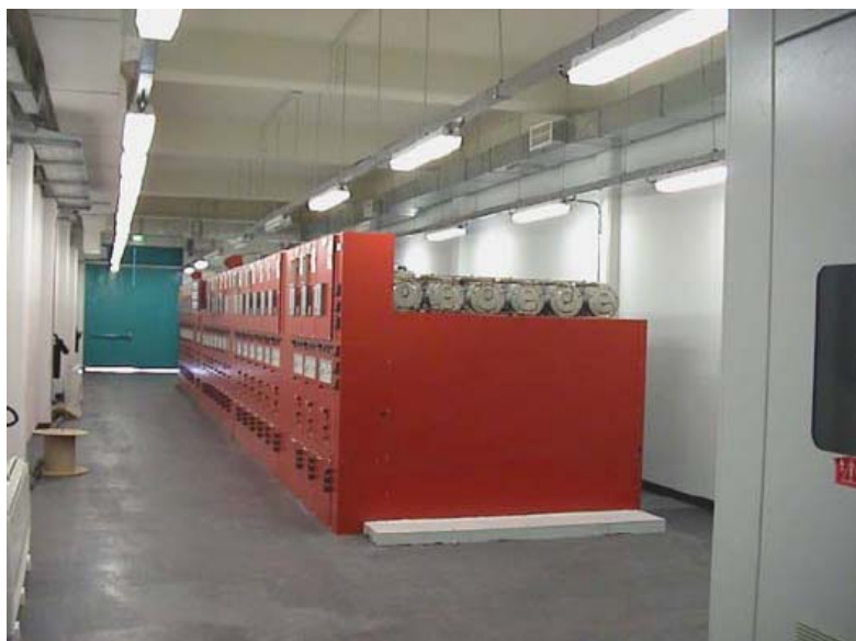
Fig. 2 33 kV 8DB GIS, with CBs protected and controlled by 7SJ63
