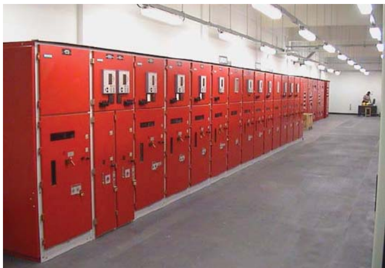
Fig. 3 6.6 kV 8BK AIS, with CBs protected and controlled by 7SJ63
