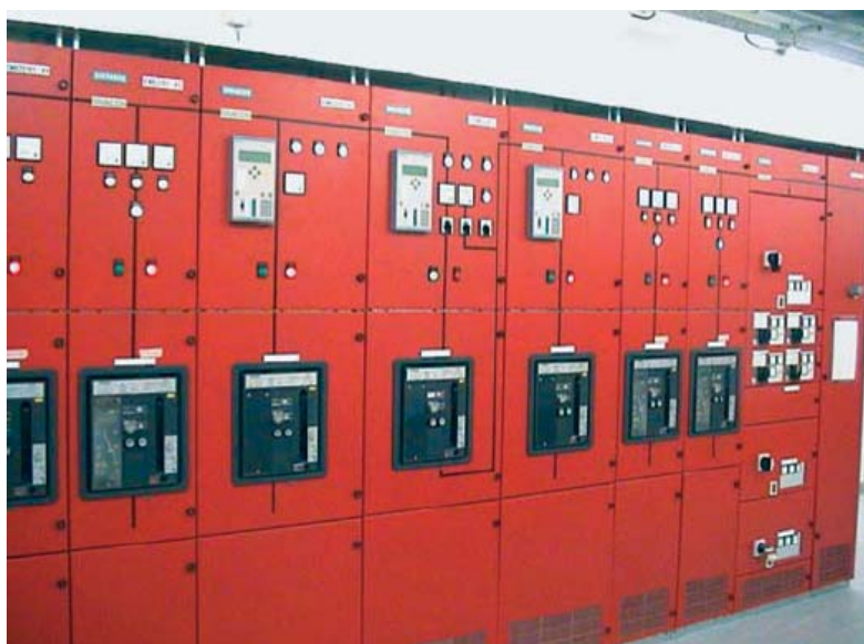
Fig. 4 400 V SIVACON, with CBs protected and controlled by 7SJ62
