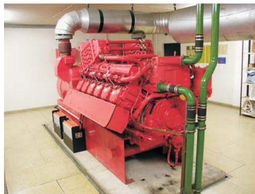
Fig. 2 Diesel generator at DEVK
