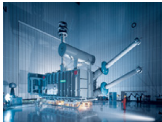
500 kV HVDC Transformer
