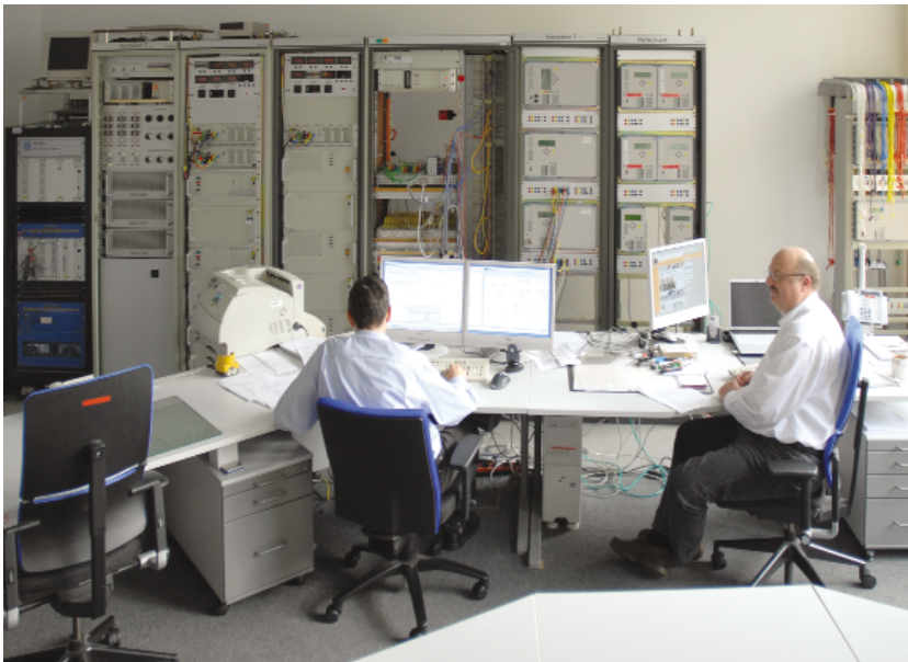
The technical equipment of the simulator with RTDS, amplifier, signal distributor and protective devices (from left to right)
