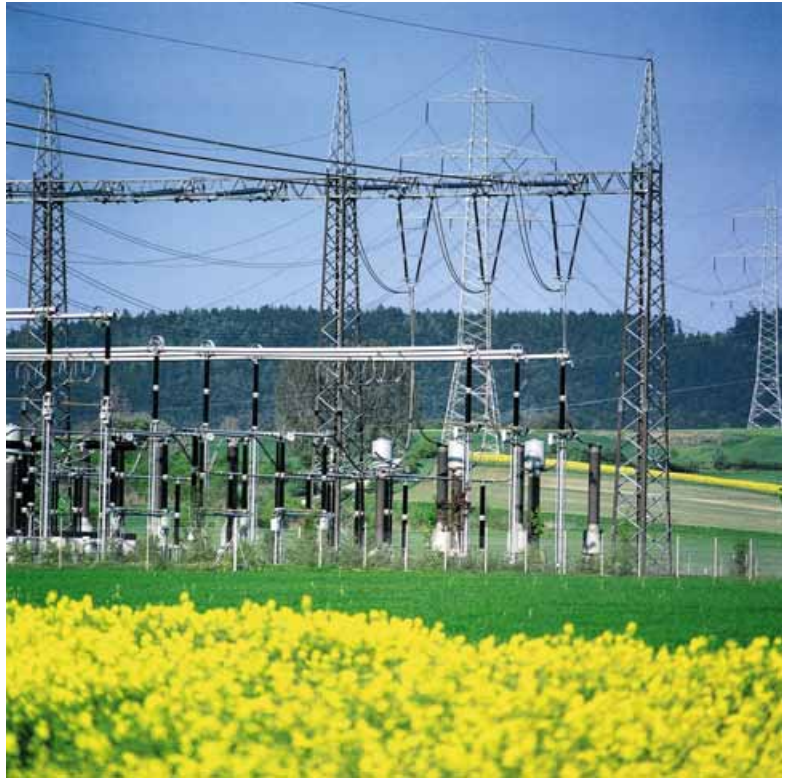
Fig. 26 400 kV outdoor switchgear
