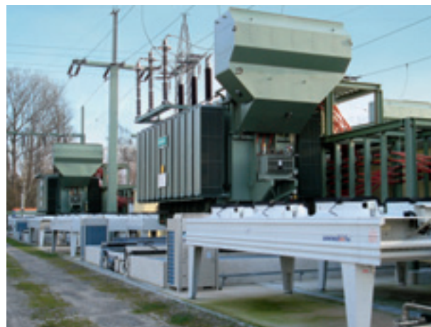
Line feeder transformer
