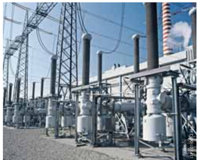
Fig. 1/16 Application in a high-voltage power system
