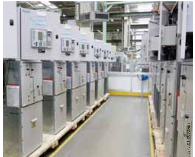
Fig. 1/3 Application in medium voltage
